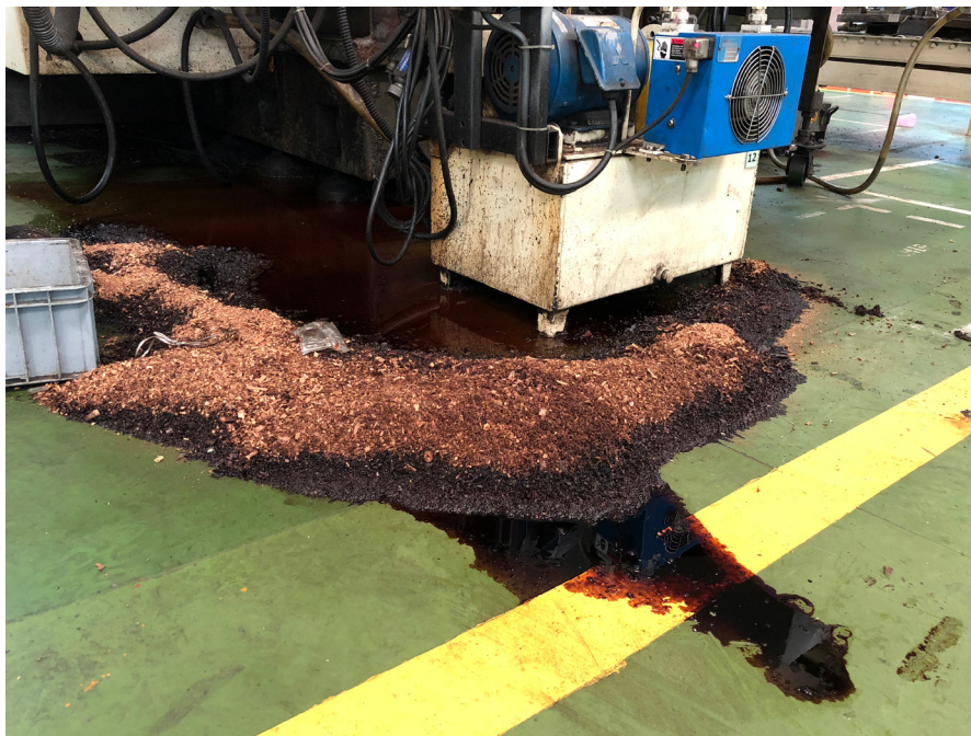
Figure 3. Hydraulic systems use various types of fluid that can be messy, slippery and hazardous to humans and the environment. As hydraulic fluids lose effectiveness over time, special care and regular maintenance is critical.
